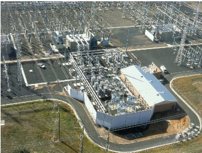
Figure 4: Armidale SVC – TransGrid
